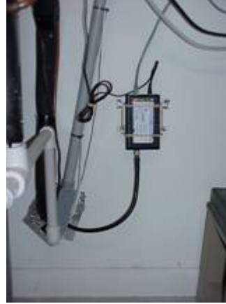
Closeup of AvaLAN Radio Installation
